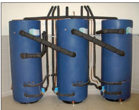
Hot water cylinders
