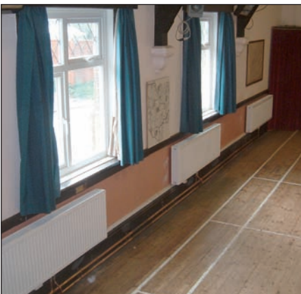
Radiators inside the hall
